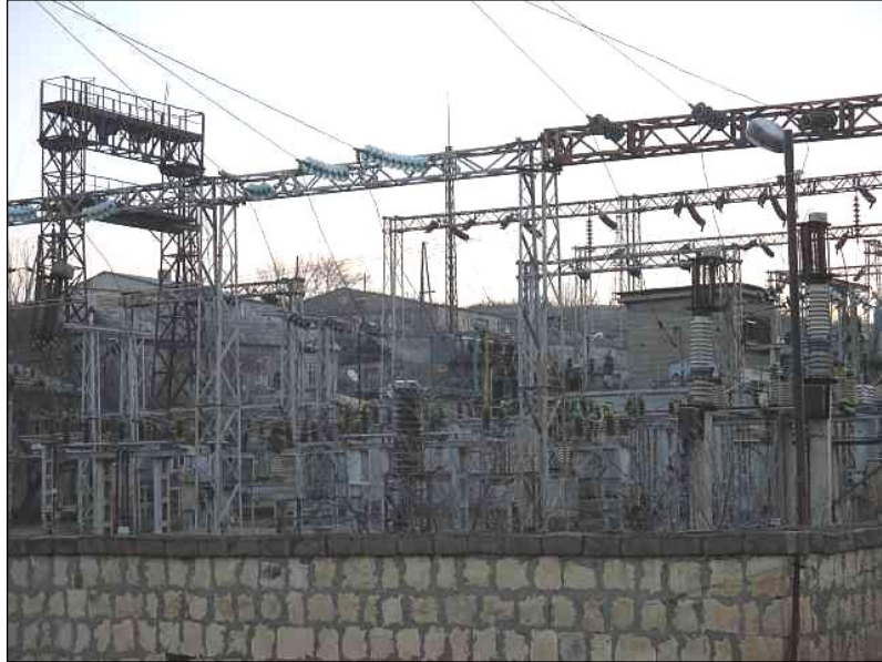
Photo 2-2: Substation Noyemberyan at Haghtanak village
