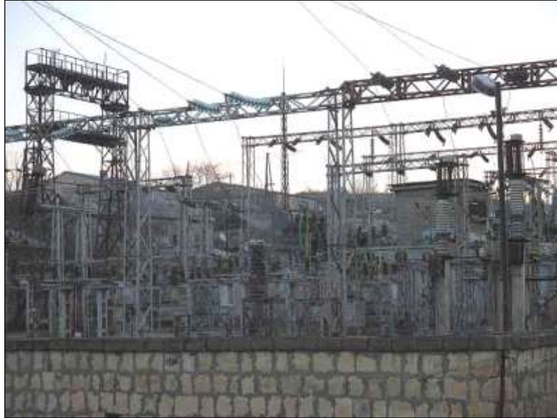
Photo 2-2: Substation Noyemberyan at Haghtanak village
